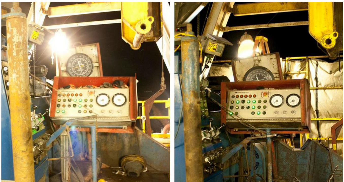
Figure 10—The shielded light at the right reduces glare and improves visibility of the console.
