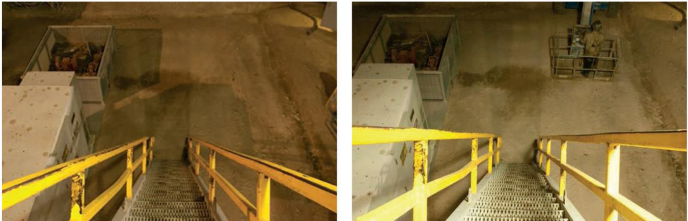
Figure 11—Before shielding, the left photo shows that the light fades toward the bottom of the stairs. The photo at the right shows well-lit stairs all the way down.
