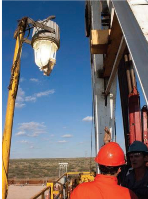
Figure 7—Workers discussing makeshift glare shields on a “360” fixture
