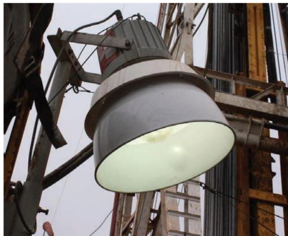
Figure 8—A “360” fixture fitted with a deep shield, which works well at greater mounting heights over stairs
